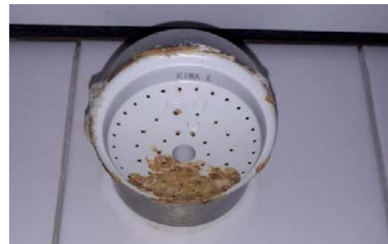
Foto 3: Point of use filter.
