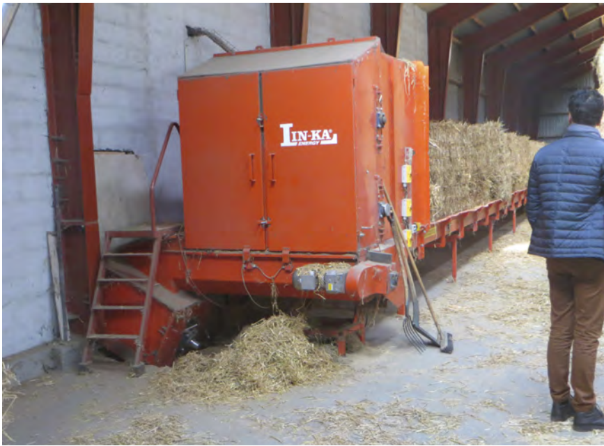
Brandstoftoevoer stro-gestookte ketels
