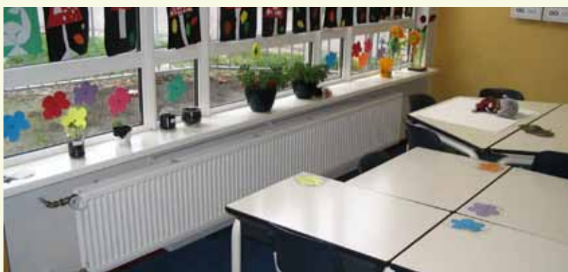
-Figuur 3- Climarad in schoollokaal (WTW)
