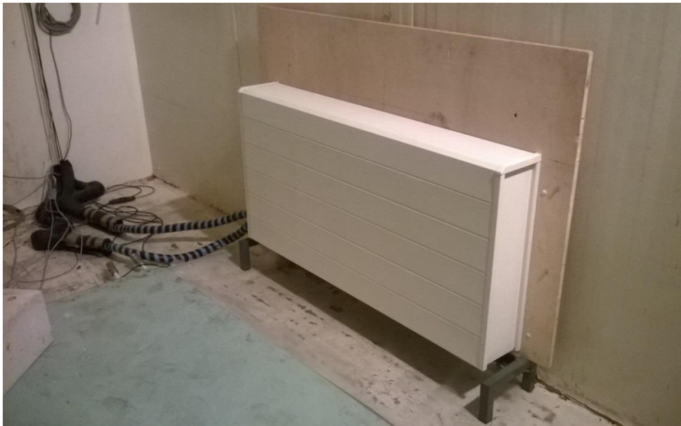
Foto 2.4 Low-H 2 O radiator in de proefkamer
